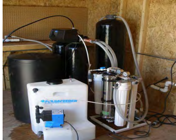
Example of a reverse osmosis system installed in the San Antonio del Desierto Mobile Home Park by Pueblo Unido Community Development Corporation for the STAT Project.
